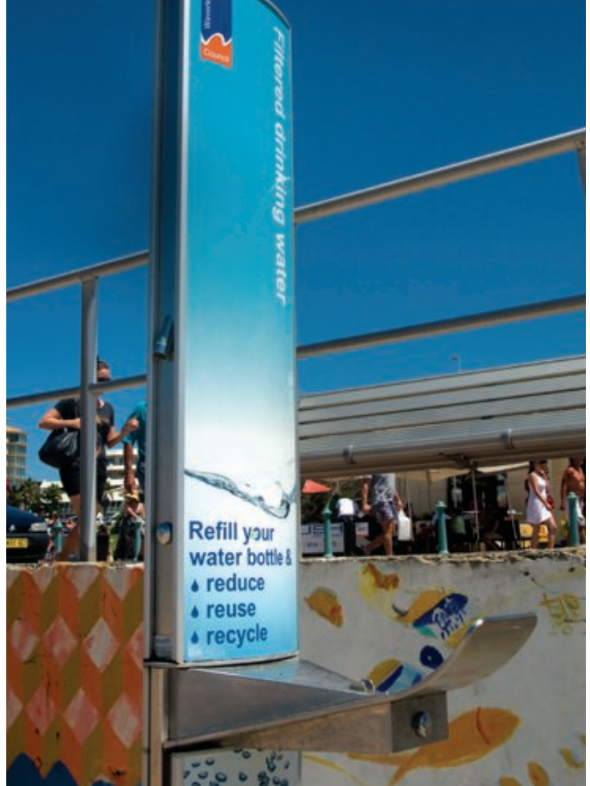
Bondi municipality has installed water stations all along the boardwalk of its famous beach.
